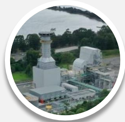
TALLAWARRA POWER PLANT - AUSTRALIA
