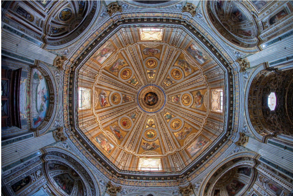
Restoration of the dome of the Santa Maria di Loreto Church in Rome @Webuild Image Library
